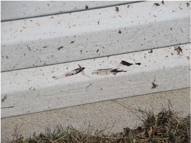
Damaged siding at pool mechanical equipment building
