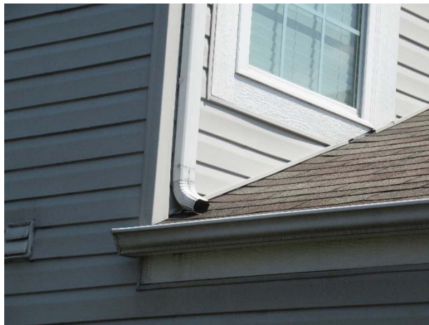
Downspout discharges directly onto roof
