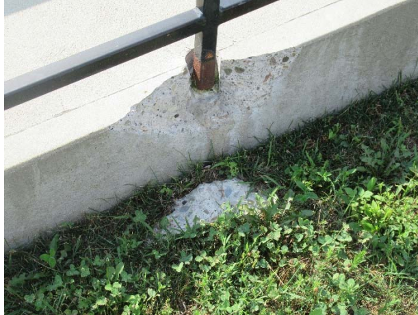
Damaged concrete at clubhouse
