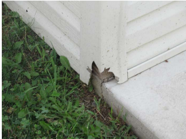
Damaged trim at pool mechanical equipment building
